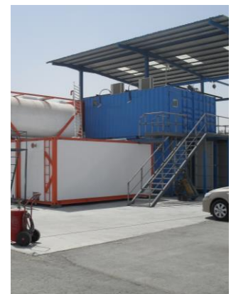
Fresh & waste water are buffered in containers
