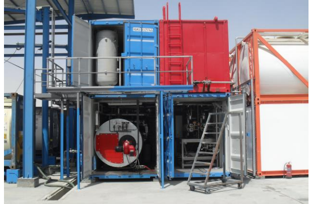
All systems are containerised
