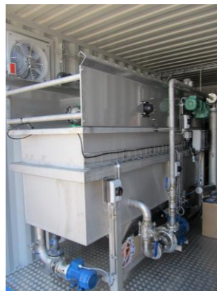
Waste water treatment
